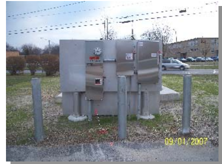
Beverly Pump Station
