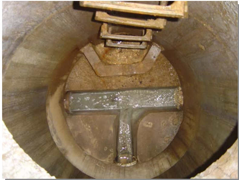
Overflow to be Eliminated
