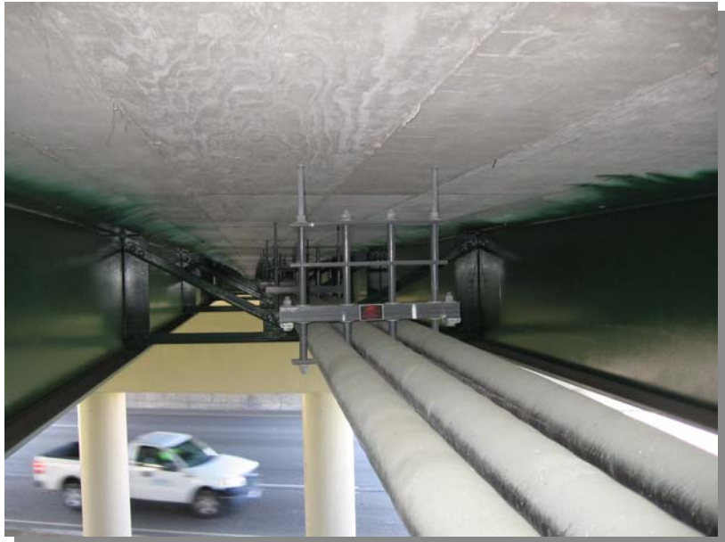
SUM-277-0247 Utility Supports
